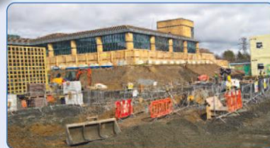
▲ DECANT WORKS AND SERVICE DIVERSIONS UNDERWAY AT THE PAEDIATRIC OUTPATIENT AND URGENT CARE CENTRE AT TALLAGHT
